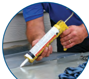
Extra Caulk & Weatherstripping
